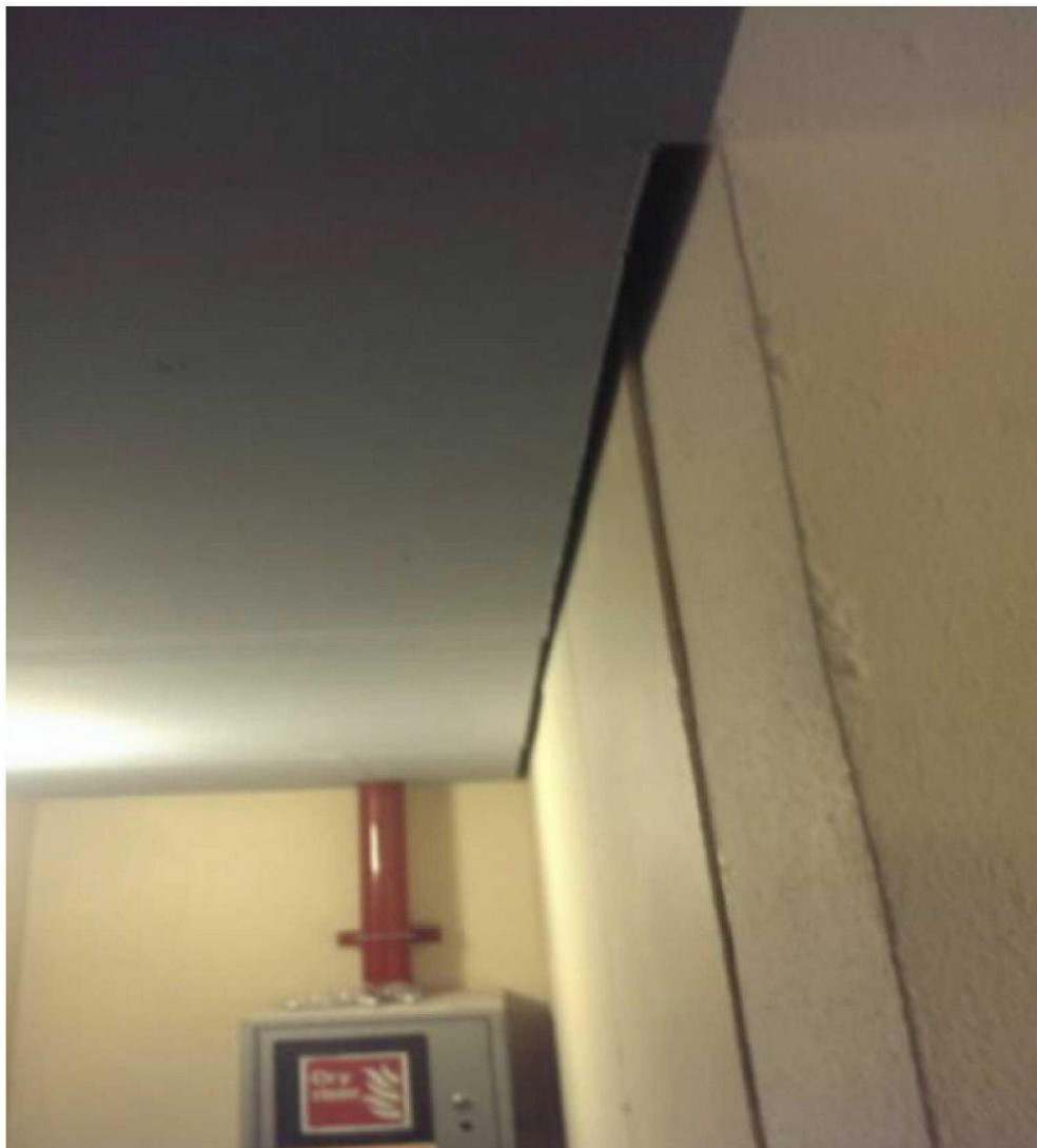
Figure 4.37: Wall access panels to be cut at new ceiling height so access to the electrical cable risers can be maintained (CST00000170)
