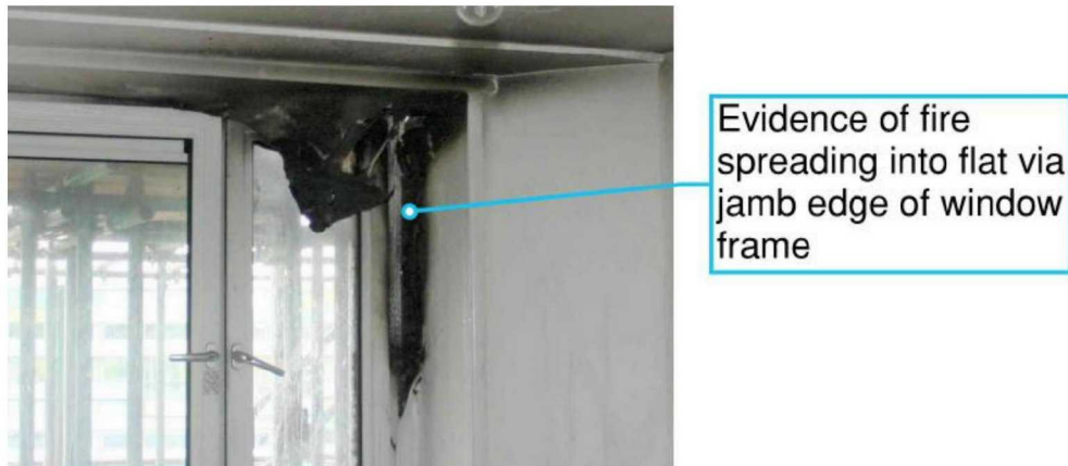
Figure 9.29: Fire spreading into flat from outside (Flat 15 bedroom)
