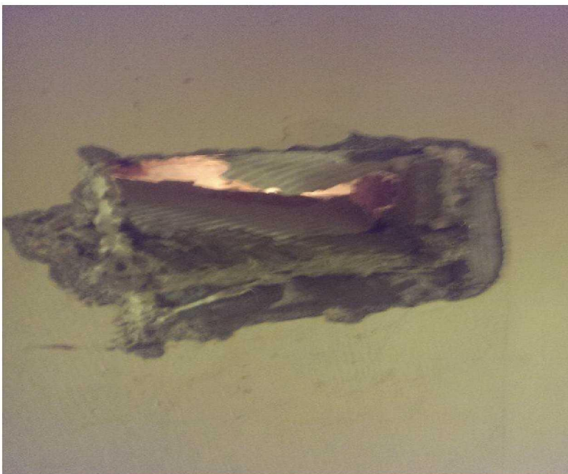
Hole in the staircase wall
