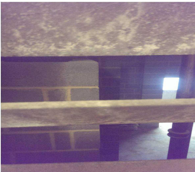
New internal construction seen on the other side of the louvered staircase vent
