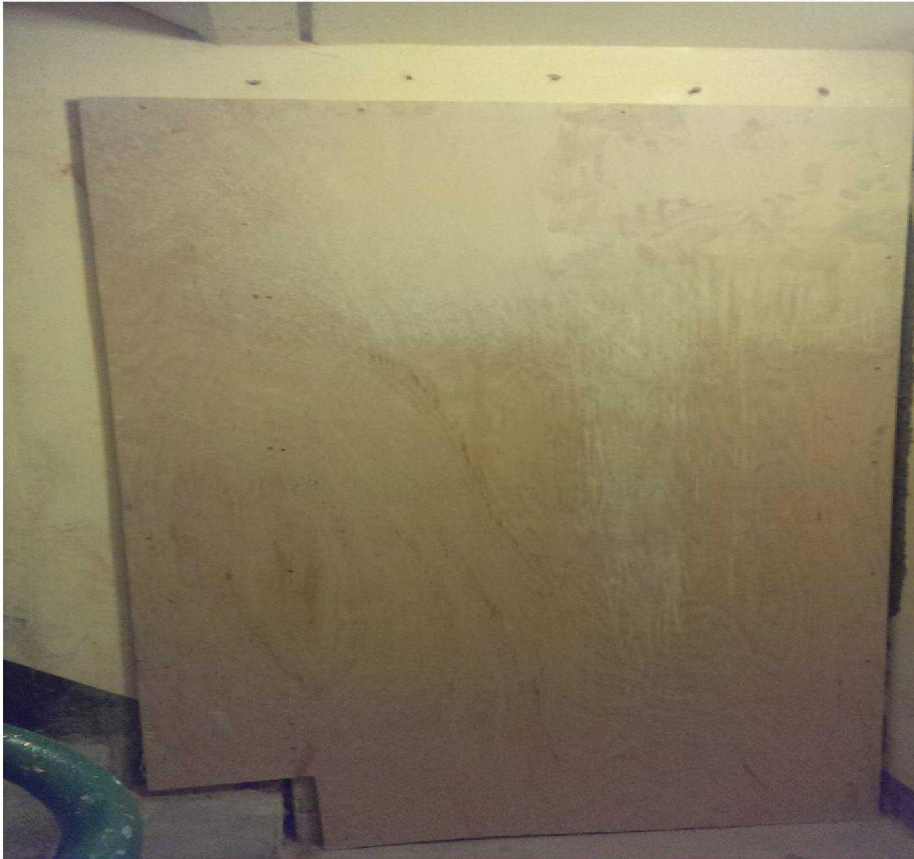
Non fire rated hoarding and a gap on the right hand side
