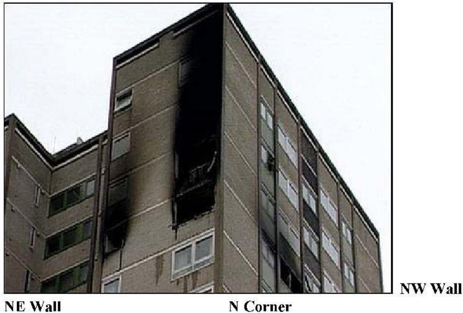
Fig 7 – Wind gusts to an estimated 23mph entered the window on the NW wall (bedroom one) to increase the burning efficiency of the fire. This wind created a very intense fire in the flat and forced a large quantity of the flaming combustion products out via the two windows on the NW wall.
