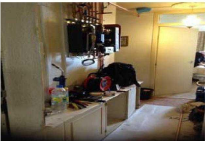
Flat 55 mechanical internal installation HIU is being installed, floor protection has been fitted.
