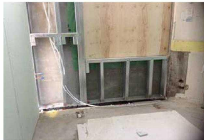
Walkway +1 can Rydons confirm that no insulation is due to be fitted between the internal and external wall void. This seems like a possible cold spot?
