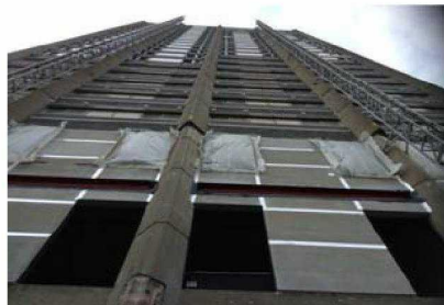
North Elevation the window frames have come down on average 14 floors down from the top.
