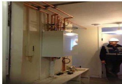
Flat 115 mechanical internal installation HIU has been installed.
