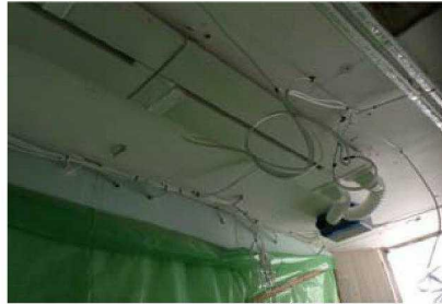
The ceiling ductwork to the HIU heating needs to be insulated to stop condensation.
