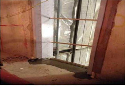
Liteg mix being mixed up to make good around inside the lift frames.
