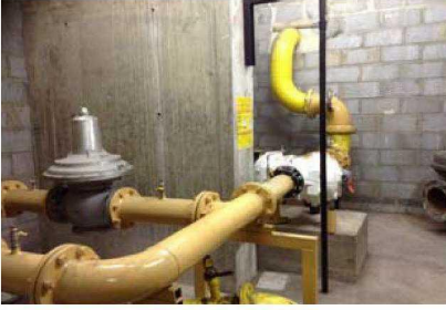
The boiler gas intake room in the basement showing the pipework that was leaking gas, that appears to have been repaired. KCTMO to confirm if this has happened.
