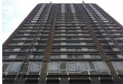
West Elevation window have now started with 12 floors frames down on the outside elevations, and down 7 floors on the middle elevation.
