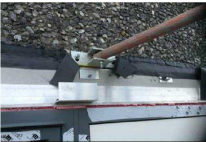
The DPC needs to be finished when the external hoist brackets are removed, the C of Works requires this to be inspected.
