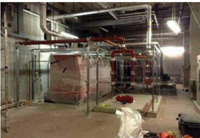
In the Basement plant room, the new three boilers and heat exchange plant are beginning to be installed, with the pipework and framing works being installed.
