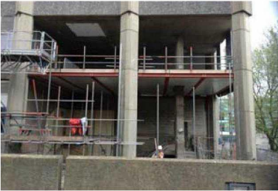
South Elevation birdcage scaffold and the concrete slab has now been poured. Works below to follow.
