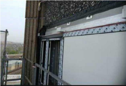
The external cladding and windows will ALL need to be inspected, checking the frames, mastic, and the works around
