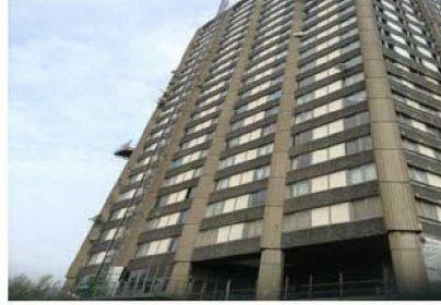
South Elevation one side of the climbing mast has been erected only. The other side has yet to start. No cladding brackets or windows have yet started.
