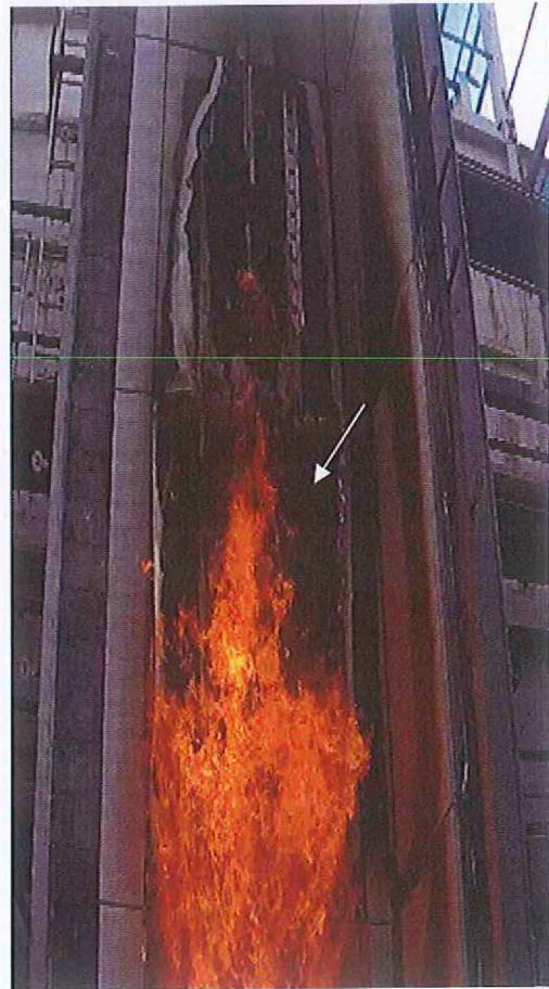
DLP C2753C/0006 M4 & M5 panels consumed by fire
