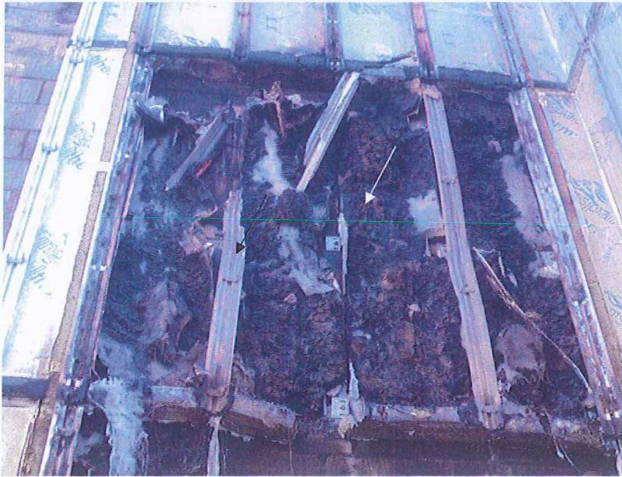
DLP C2753C/0009 Burned Kooltherm K15 insulation and railings
