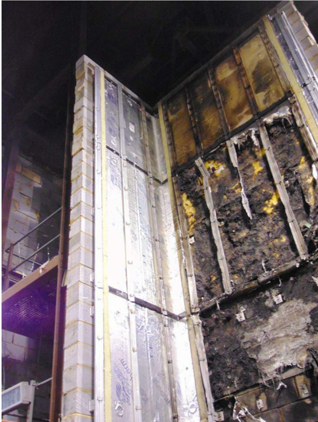
Figure 21. Aluminium rail substructure and thermal insulation following removal of ACM panels (wing wall, approximately 1300mm-6500mm above the combustion chamber).
