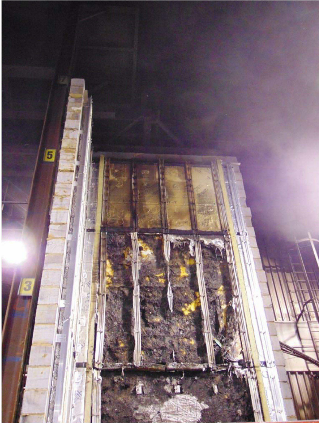
Figure 20. Aluminium rail substructure and thermal insulation following removal of ACM panels (main wall, approximately 1800mm-6500mm above the combustion chamber).
