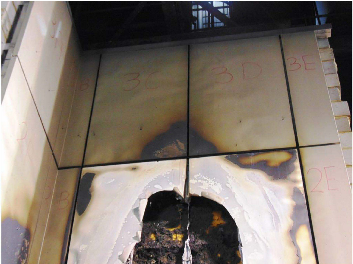
Figure 19. Row 3 post-test (main and wing wall, approximately 4600mm – 6500mm above combustion chamber).
