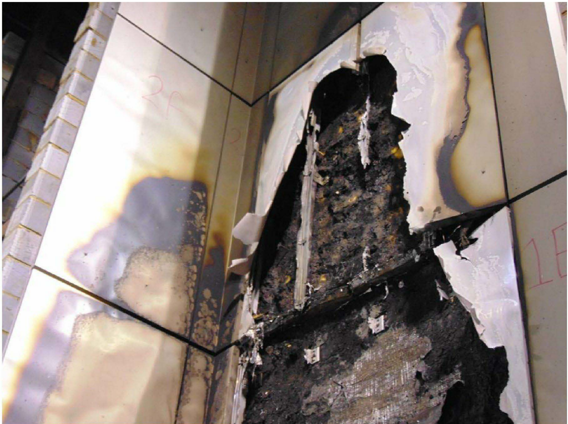
Figure 18. Row 2 post-test (main and wing wall, approximately 2300mm –4600mm above combustion chamber).
