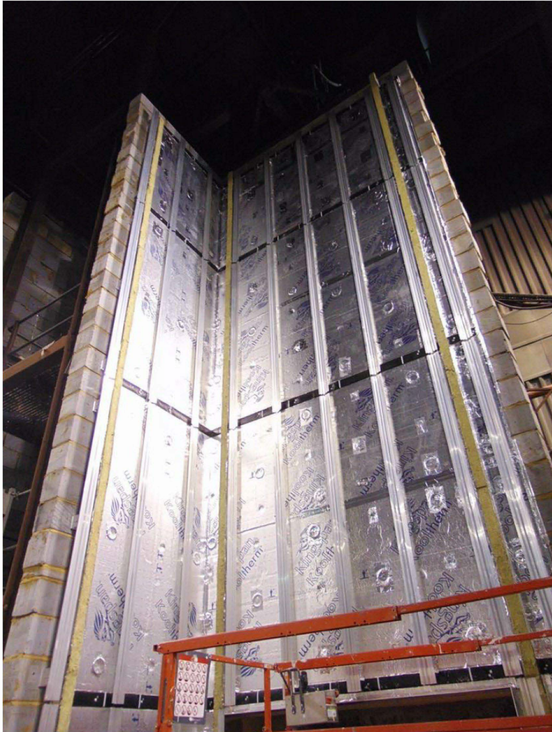
Figure 6. Aluminium substructure, cavity barriers (horizontal and vertical) and thermal insulation installed on the system.
