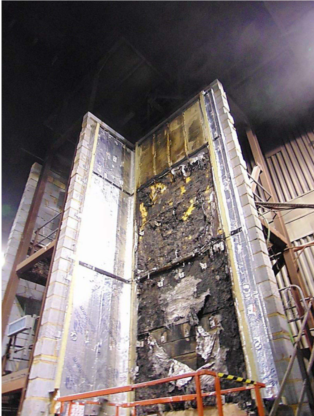
Figure 22. Thermal insulation following removal of ACM panels and aluminium substructure on the main and wing wall (approximately 200mm – 6500mm above combustion chamber).
