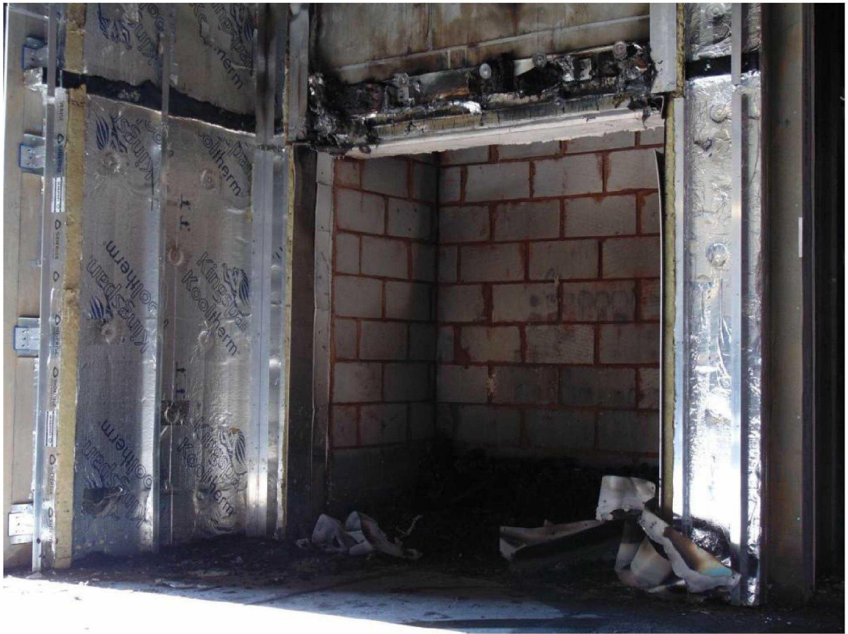
Figure 26. Damage to insulation between ground and top of combustion chamber opening.
