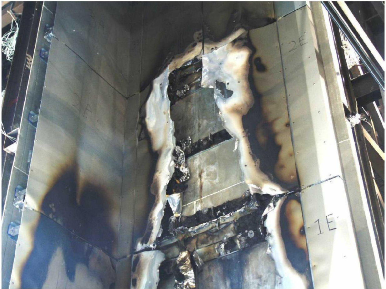
Figure 23. Damage to panels between a height of approximately 4000mm and 6000mm above the top of the combustion chamber.
