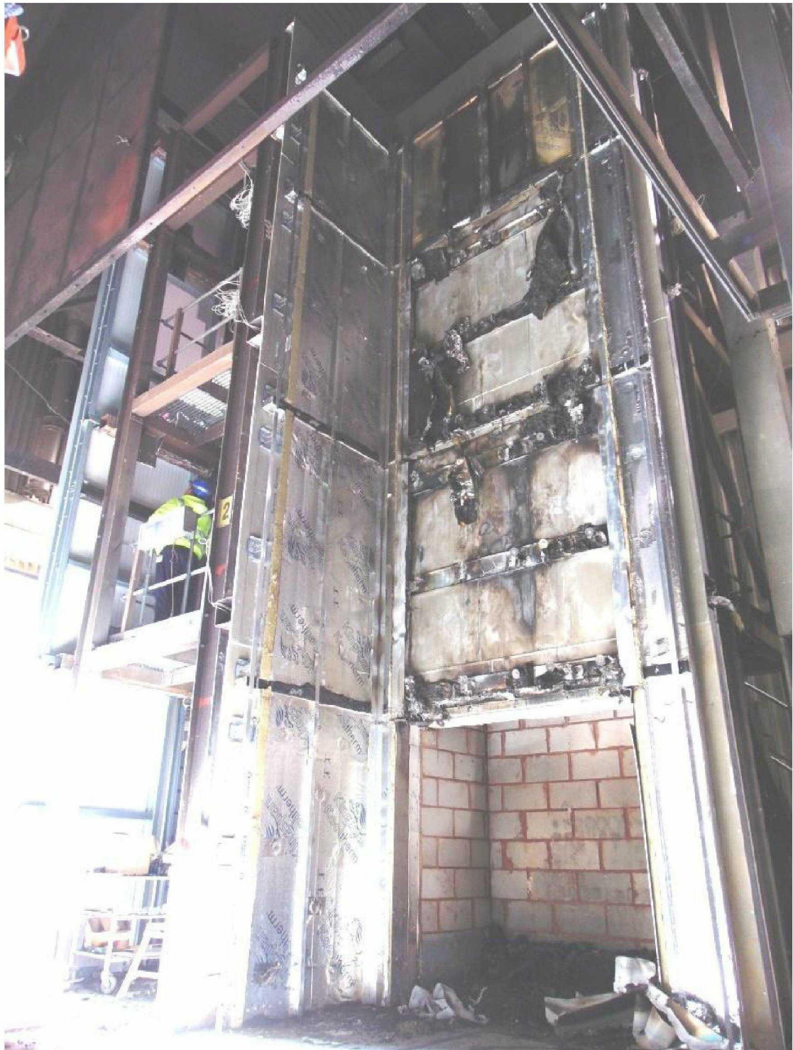
Figure 25. Full-height photograph of damage to insulation.
