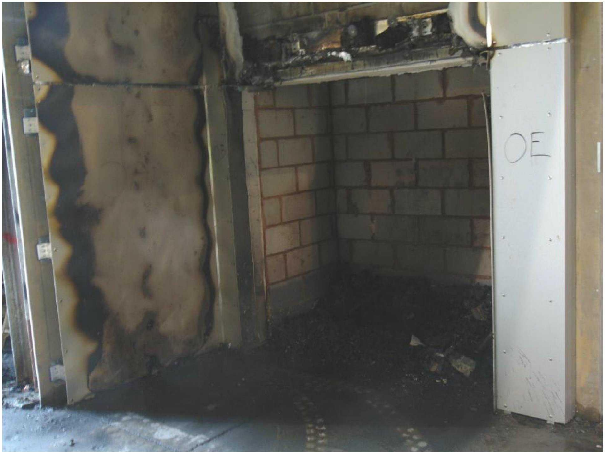
Figure 21. Damage to panels between ground and top of combustion chamber opening.
