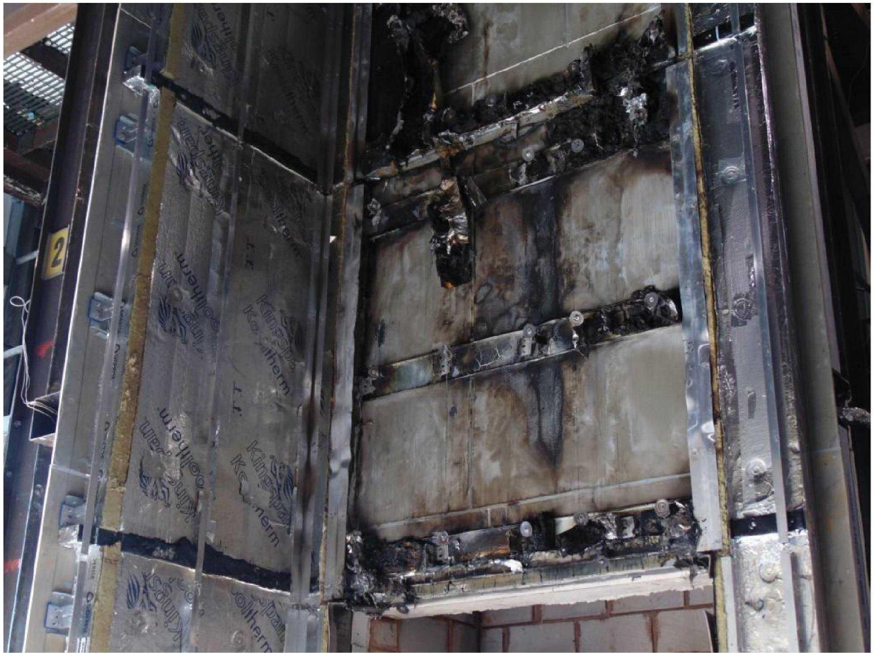
Figure 27. Damage to insulation between top of combustion chamber and a height of approximately 4500mm above the top of the combustion chamber.
