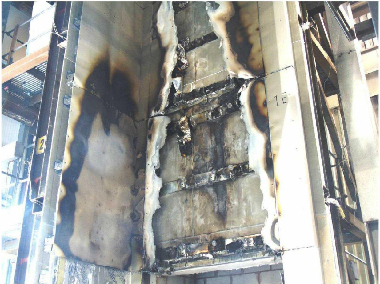
Figure 22. Damage to panels between top of combustion chamber and a height of approximately 5000mm above the top of the combustion chamber.
