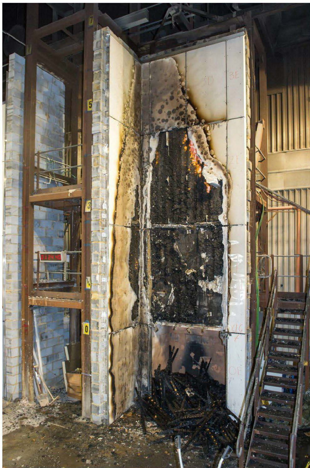
Figure 22. Full height photograph of system post-test – general.
