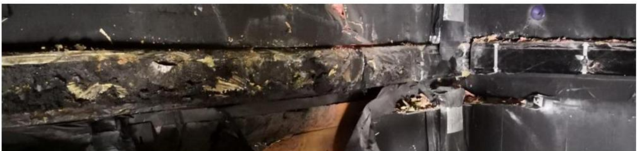
Figure 4.22. Post-examination damage. Photo of the middle horizontal fire barrier installed on both faces. Partially activated on the main face but in-place; not activated or detached on the wing face.
