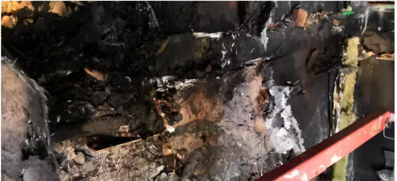
Figure 4.20. Post-examination damage. Photo of the bottom horizontal fire barrier installed on the main face. Fully activated and partially detached (especially above the chamber).
