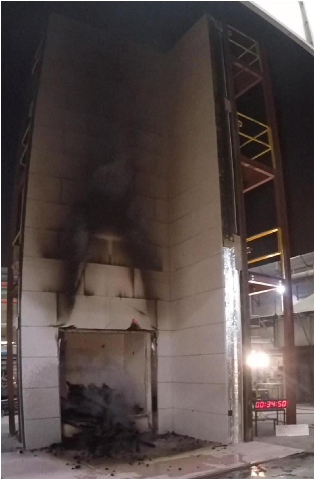
Figure 4.13. Cladding system after fire extinguishment (34 min 50 sec after ignition of the crib).
