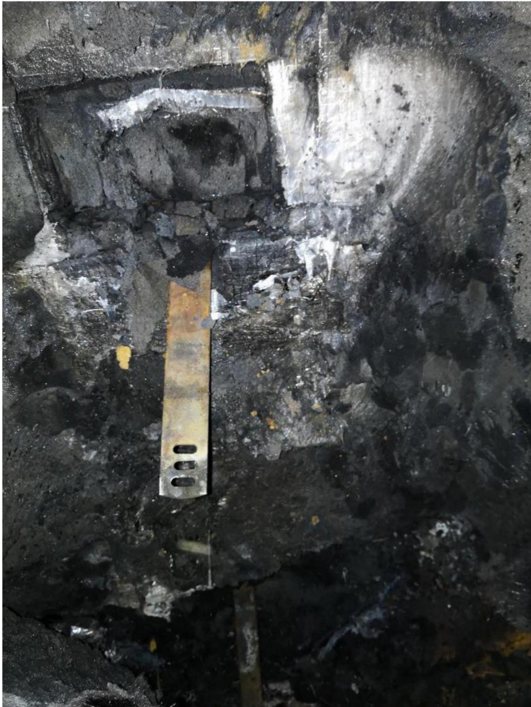
Figure 4.23. Post-examination damage. Photo of one bracket located just above the combustion chamber. No damage except discoloration observed.
