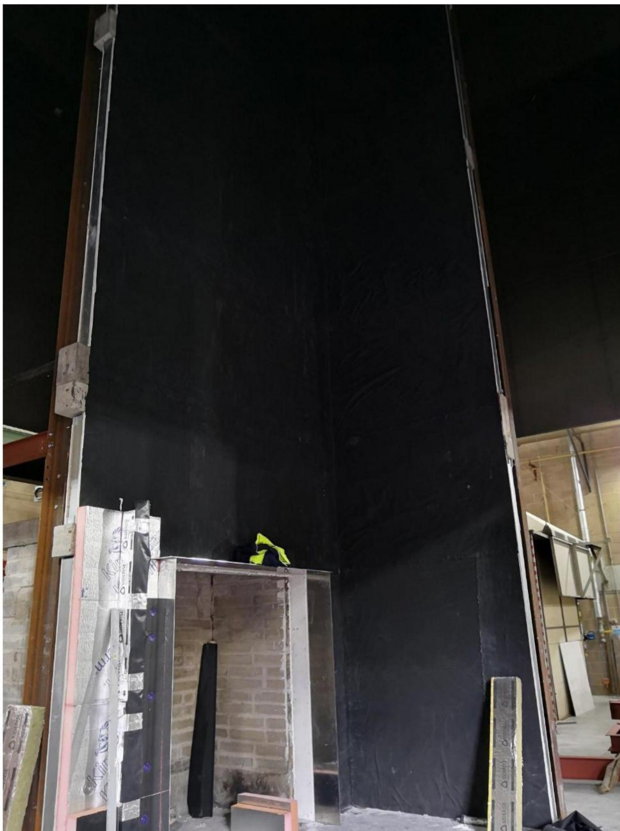
Figure 4.5. Installation of waterproof membrane completed during construction. Aluminum pod-frame also shown. Start of insulation and vertical fire stop barriers installation.
