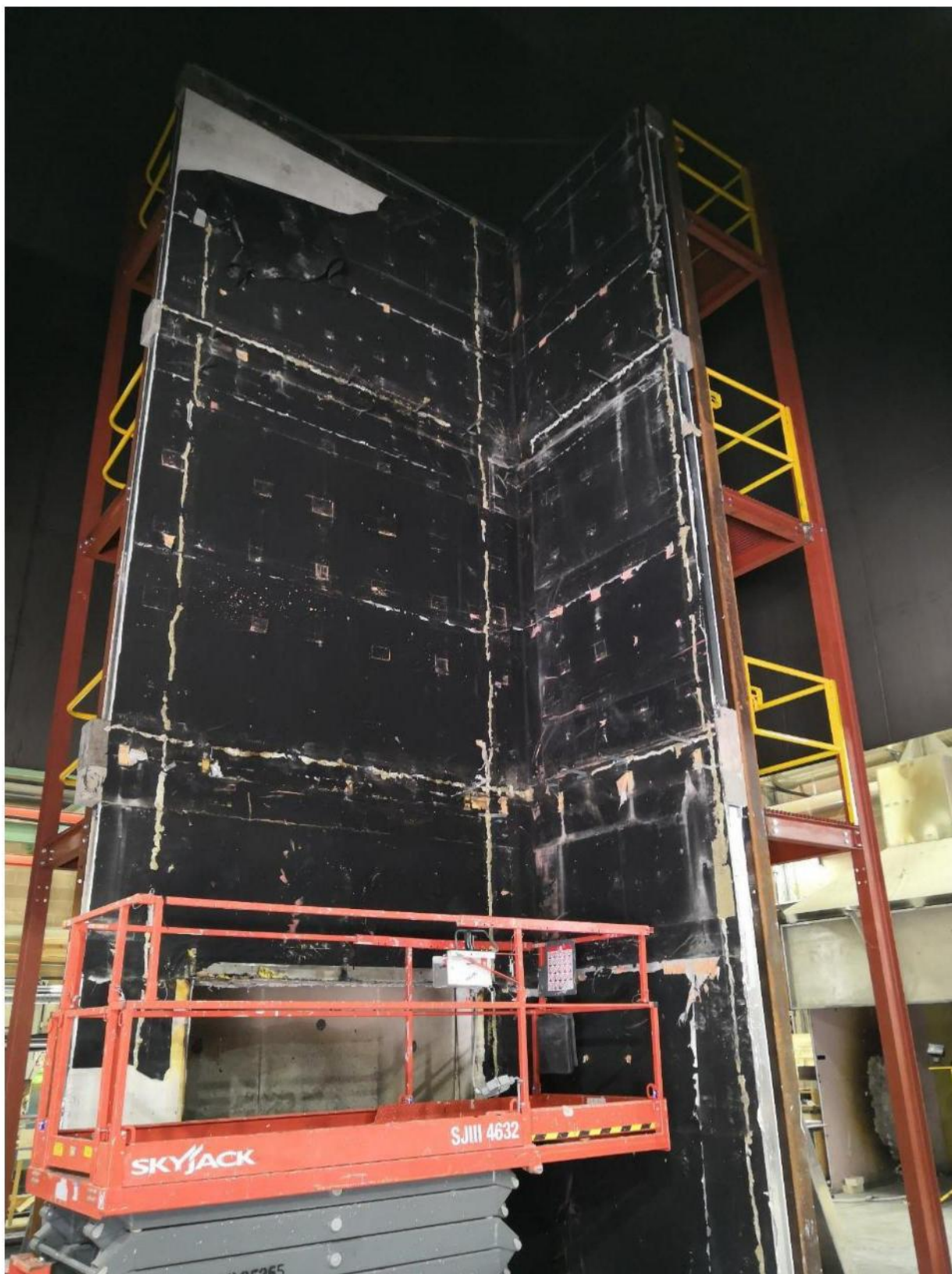
Figure 4.24. Post-examination damage. Waterproof membrane intact and in place after removing insulation layer from system.
