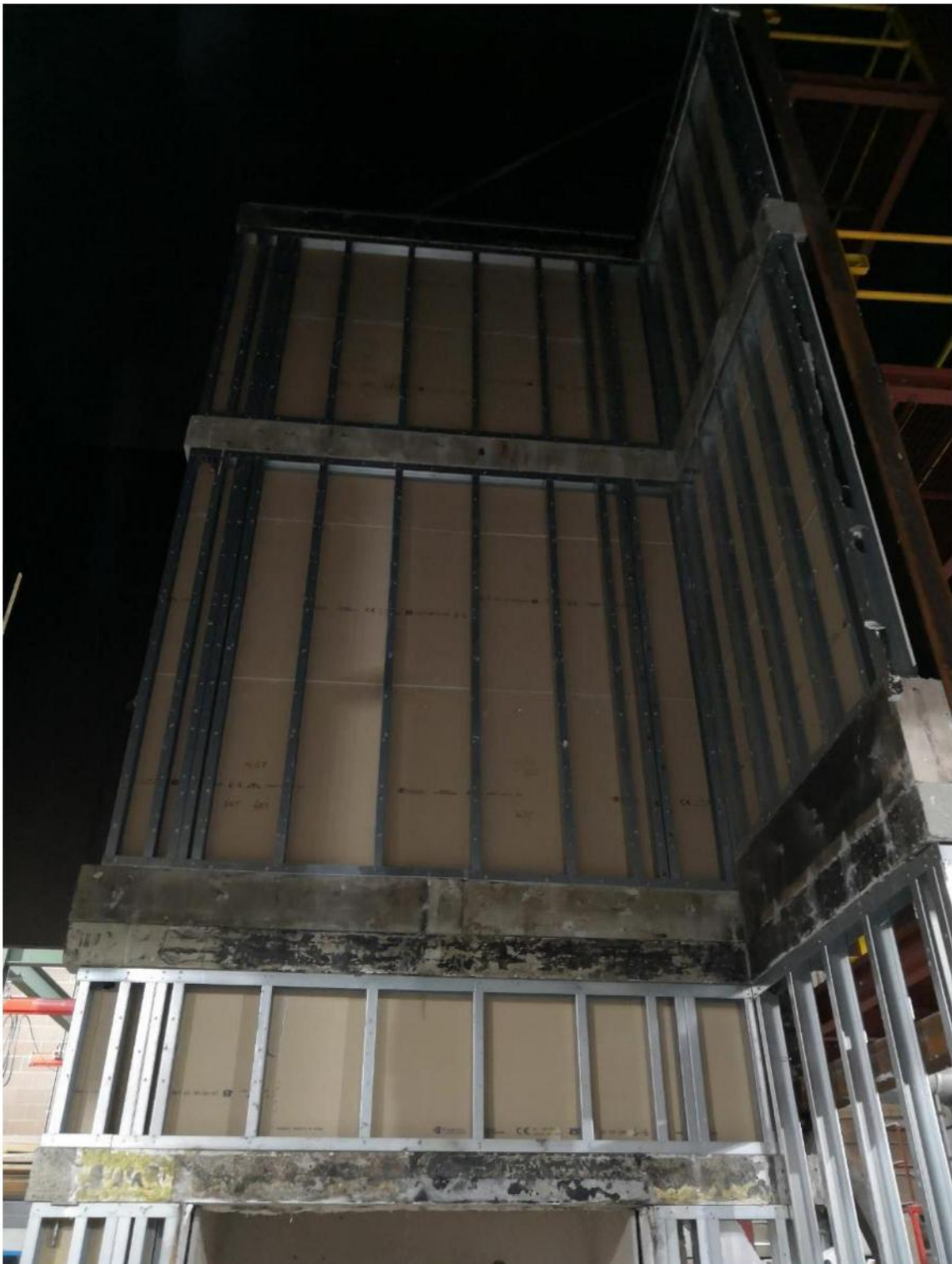
Figure 4.25. Post-examination damage. Photo of the system showing the plasterboard layer and SFS Kingframe after the test.
