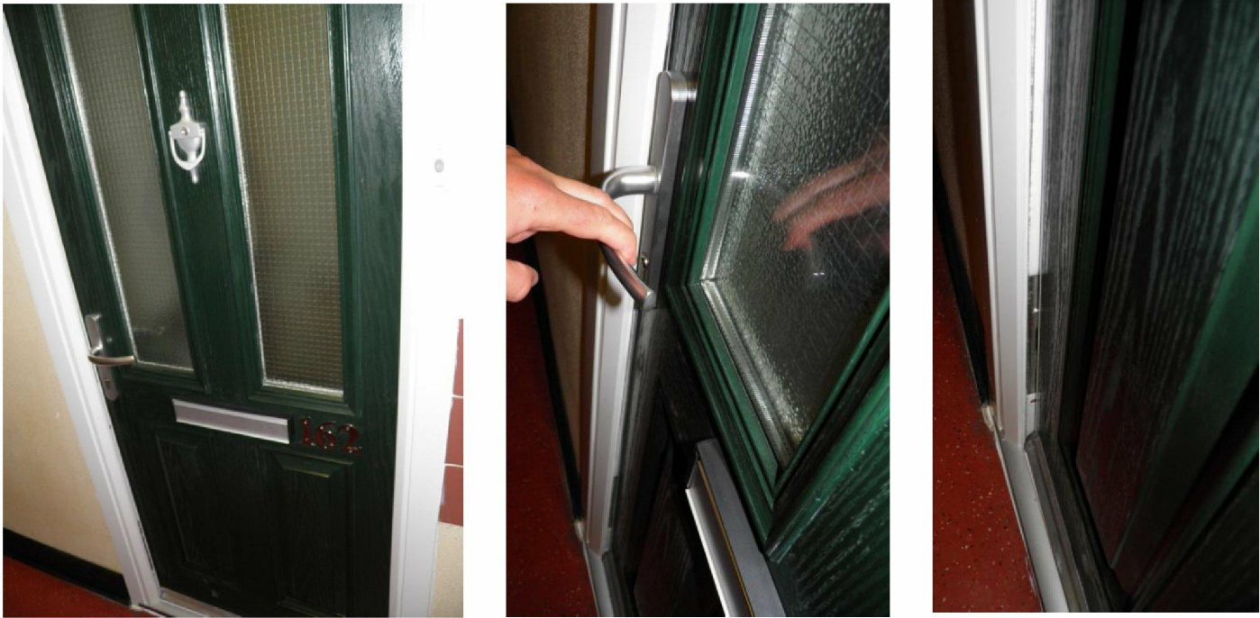
Flat 162 at Grenfell Tower where resident experienced problem with closing this door due to door/frame was fitted out of plumb.
