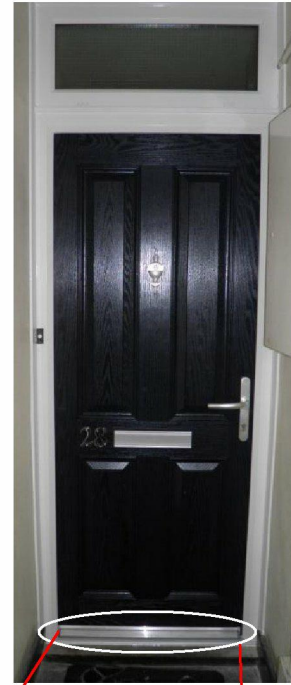
This image illustrates that drip detail was fitted off centre.
