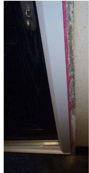
Frame was fully foamed and fitter was instructed to place packers in.
