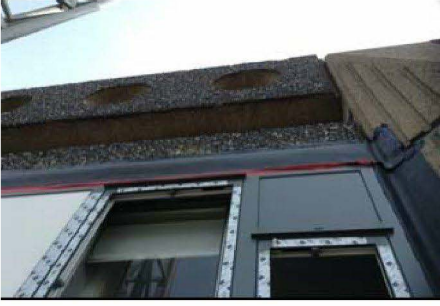
Rydons are proceeding now with the original tendered design, for the cladding parapet detail.
