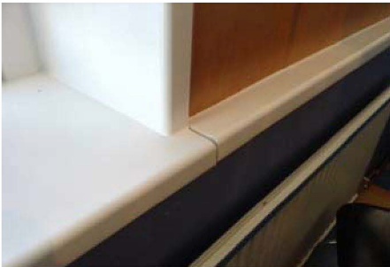
Flat 101 has just been installed, but the trims are missing. Please fit asp.
