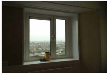
Flat 145, internal window trimming has been finished and KCTMO has agreed the finish. As from today 9 flats have been finished, including old frames out, new glass and trims fitted.
