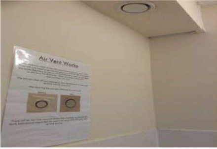
A total of 63 no off existing bathroom and WC ventilation ducts have been cleaned and new cover has been fitted.
