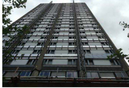
North Elevation the window frames have come down all the way to 20 floors down from the top. Bottom brackets have now started to be fitted, and gazing to the walkway + 1 level has also been finished, and infill panel to one section between the 1st and 2nd floor has been fitted.
