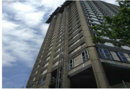
South Elevation both of the climbing masts are in use. The setting out has started, and the brackets has started Monday 15th June.
