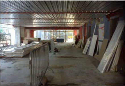
The ground floor level, no partitions and no M&E has progressed yet.
