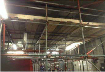
All the Birdcage scaffolding above the existing boilers has been installed, for high level new service pipes is progressing.
