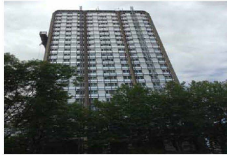
East Elevation the window frames have come down all the way to 20 floors down from the top. Bottom brackets have now started to be fitted and gazing to the walkway + 1 level has also been finished. No infill panels have started.
