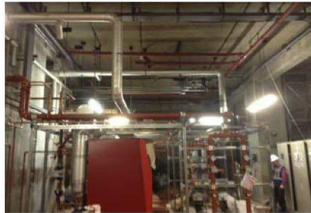
Basement high level pipes and valves, and flues have been done above the new boilers, only, and scaffolding has been dismantled.
