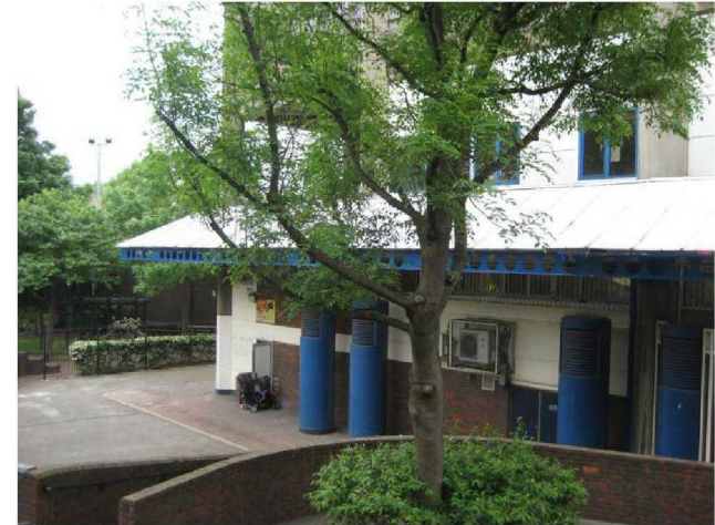
Existing external canopy fixed to the RC columns, view from the ramp
