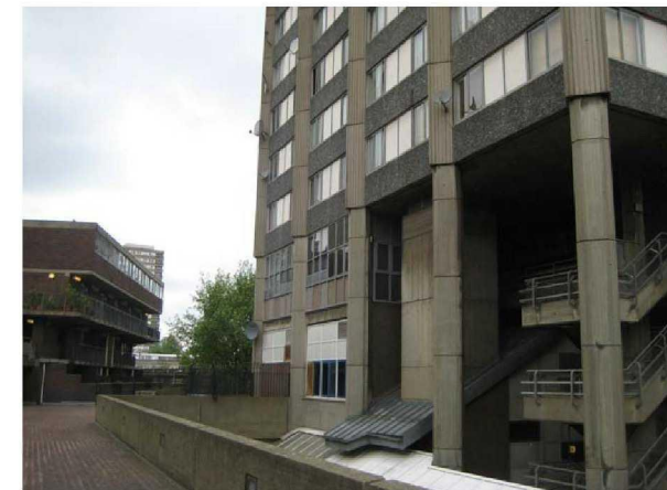
View of the existing external lift and stair, both to be demolished
