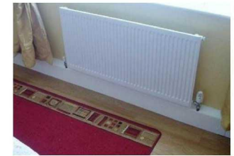
Figure 7-23 - Typical Pendock profile and radiator arrangement
