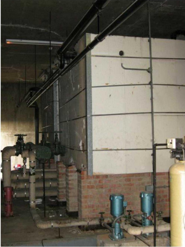
Figure 8-2 - Non-Potable Water Tanks
