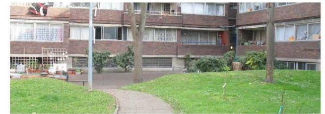
Fig. 21 Louvred vents to existing garages. Baseline windows can be seen to the right.
