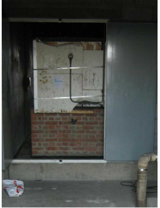
Figure 8-3 - Potable Water Tank
