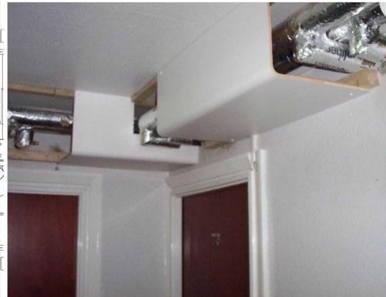
Figure 7-7 - Pendock profile boxing in high level pipework
