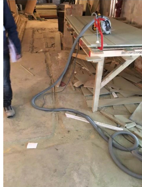
Photo 6 – Poor housekeeping / MDF dust not managed.
