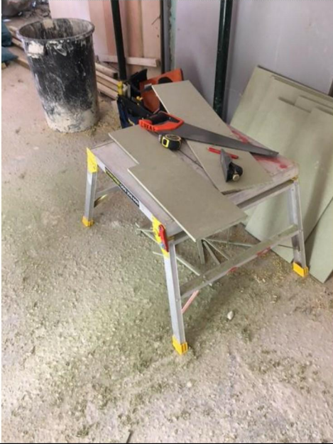
Photo 5 – working MDF – not in line with COSHH assessment
