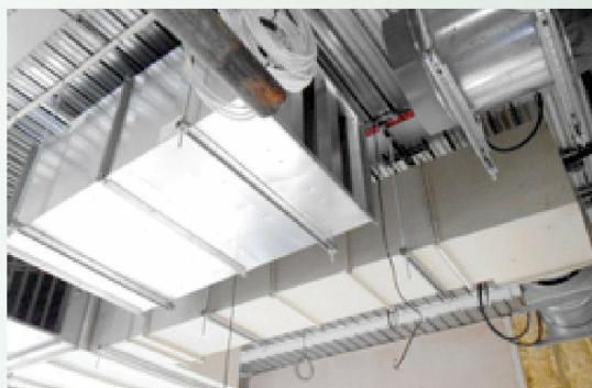
New heating and ventilation ducts in the foyer, before a false ceiling covers them
