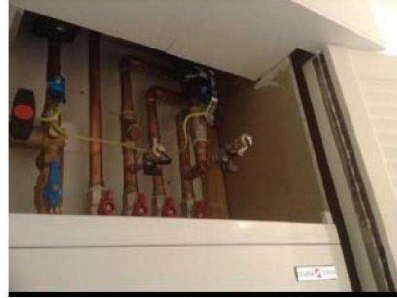
The new HIU's in the old flats have been installed with a new water mains stop cock positioned above the unit, and possibly difficult to get to for an old person. Has the position been agreed? KCTMO and Rydons to comment please.
