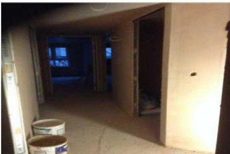
Mezzanine last flat to the South West corner, plastering now done, and 2nd fix carp and M&E to start soon.
