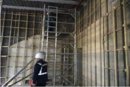
Mezzanine +1, entrance hall, battening for the cladding in progress. The AOV needs to be fitted first before all the finishing trades can be done. This should be installed according to Rydons in Six weeks.
