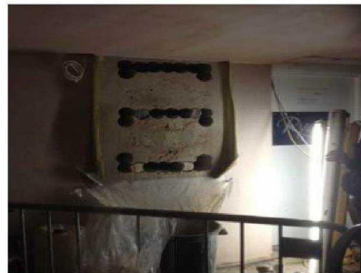
The last AOV structural openings are still being cut out, the last to be done is the Mezzanine floor.
