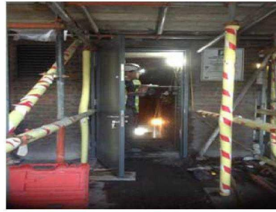
New basement plant room door is now being fitted. Rydons to make sure all parties have a key including all the KCTMO maintain acne staff.
