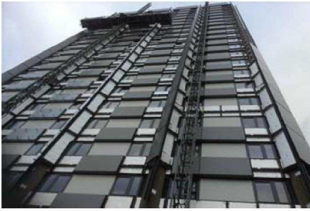
South Elevation - 138 panels out of 240 have to be fitted. 80% of the column brackets have been fitted, and the top canopy is nearly done. 30 of the 184 column panels have been fitted. Lower entrance framework is now being installed. Only one mast climbers is working with 3 operatives today.
