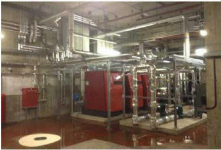
The boilers still have been commissioned, but will have to be commissioned again when the permanent ventilation fans have been fitted. Labelling of all valves, schematic layouts, and general finishing off to all plant to be done.
