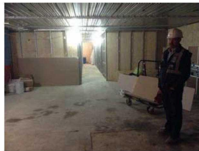
Ground floor area, and nursery area, partition have started one side, 1st fix M&E has just started.
