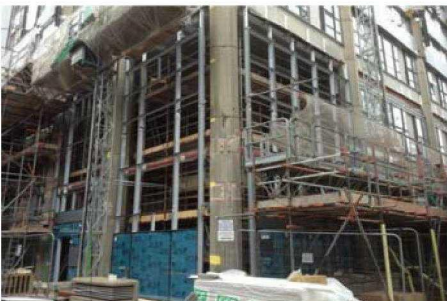
The South East corner the cladding is proceeding, and the glazed panels have also started.
