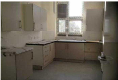
Walkway + 1, progressing well. All finishing trades are in progress, with lots of small things to be completed like the extract fans, glazing missing, etc. Still no power.
