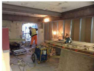
The ground floor openings are being formed, and the partitions have also started.
