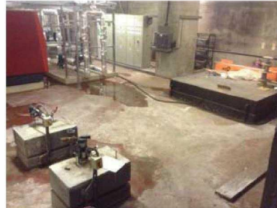
In the basement water flooding has now been resolved. Only small puddles left.
