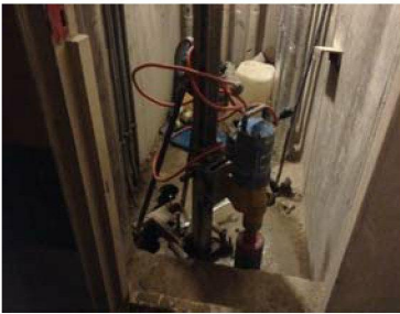
All the AOV holes are cut out except the last one being cut out today. The extract ducting is not yet on site.
