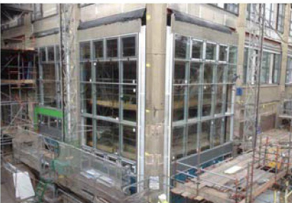
The South East corner the cladding is proceeding, and the glazed panels have nearly finished. The column trims are now being fitted.
