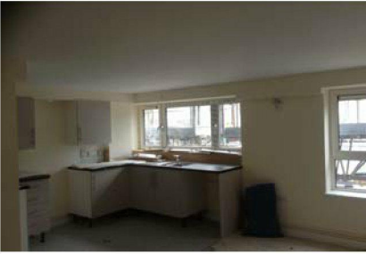
Mezzanine flats progressing well. Max Fordams and Rydons to confirm No heat or smoke detectors are scheduled to be fitted, on all of the mezzanine flats, and this has been approved by building control.
