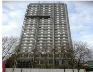
East Elevation - Still 16 panels out of 296 have to be fitted. 90% of the column brackets have been fitted, with 112 column panels fitted out of 138. (Not including the lower floors). The top canopy has nearly finished. No lower floor panels have been fitted. Snagging only to the North climber started today.
