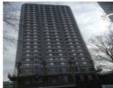
West Elevation - has been snagged and de snagged down to level 3. Both master climbers have come down to level 3. Lower floor cladding has now started.
