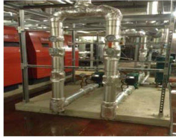
The new pipes to the basement have been lagged, and has started to be clad.
