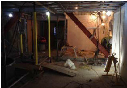
The two steel supports to the ground floor entrance hall are being fitted today.
