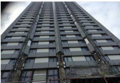
North Elevation - has been snagged and de snagged down to level 3, all finished apart from the panels around the hoist ties. Master climber has not started to come down. Lower panel have made a start.
