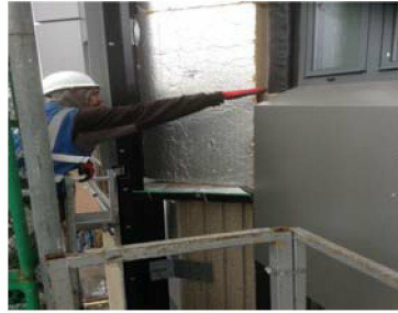
The South Elevation cannot be finished at all, because the access behind the West climber on the South Elevation, is totally unsafe. This needs to be resolved by Rydons and the cladding fixers. This has been an issue for months. This item is on the critical path.
