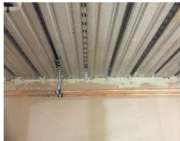
Ground floor fire seal needs to be improved before being approved, top of partition, just north of the concrete core.
