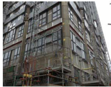
Low level cladding is progressing slowly. Picture of the North East corner.
