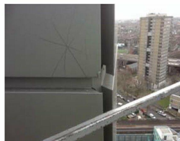
The East elevation as snagged today. A further 3 cladding panels were damaged and need replacement. A total 16 panels have needed to be replaced so far.
