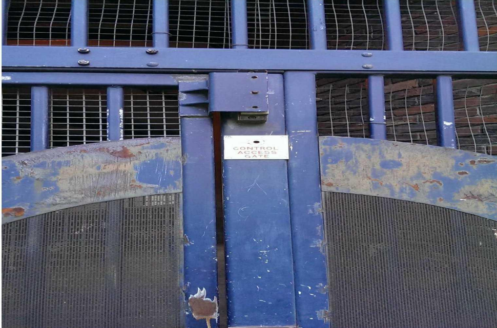
Fire fighter over ride switch fitted to pedestrian gate
